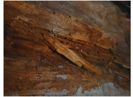
live sub-termites - framing/sheathing
