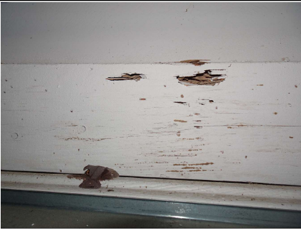
sub-termite galleries in garage
